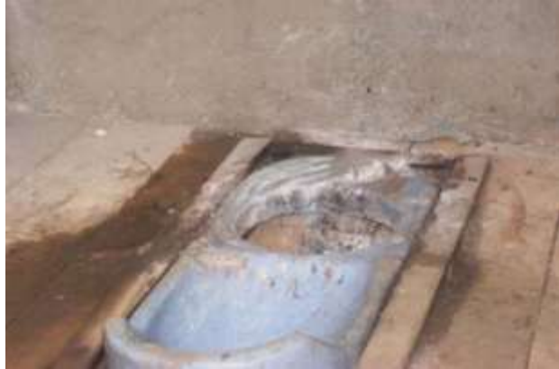
Figure 5 Eco-san toilets (after)
