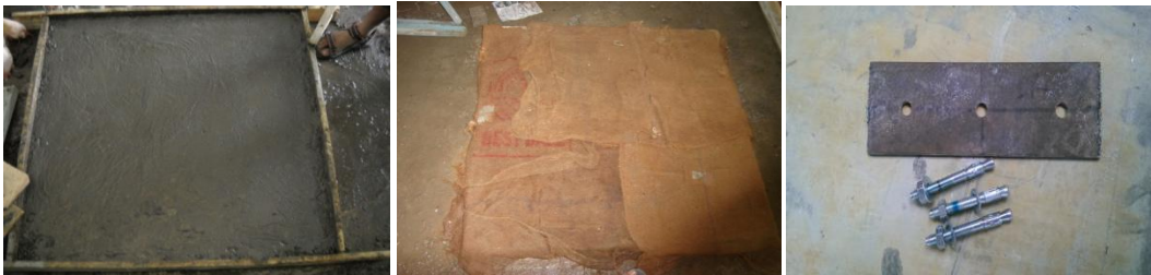
Fig.4:- Compacted concrete, curing of slab using gunny bags, and anchor bolts and plate.
