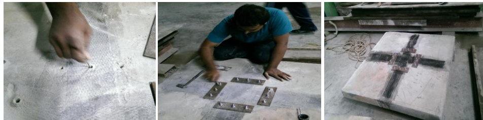
Fig.6:- Installation of anchors carried out as per previously specified steps in this project work.
