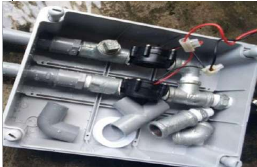
Fig. 4:- Part of pipelines and the position of mini hydroelectric.
