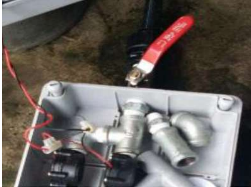
Fig. 5:- Stop clock valve view control.
