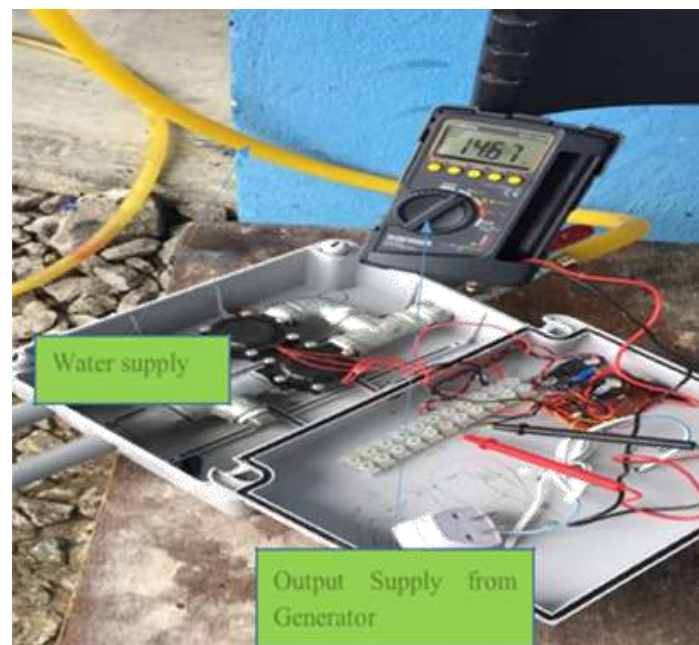
Fig. 8:- Output voltage from generator.
