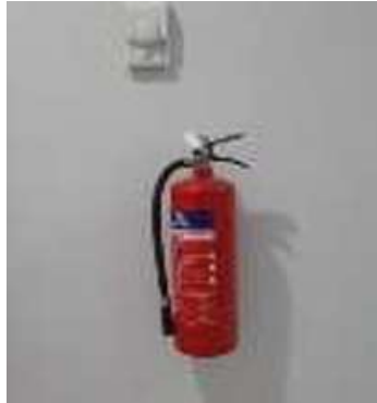
Figure 6:- APAR Protection System.
