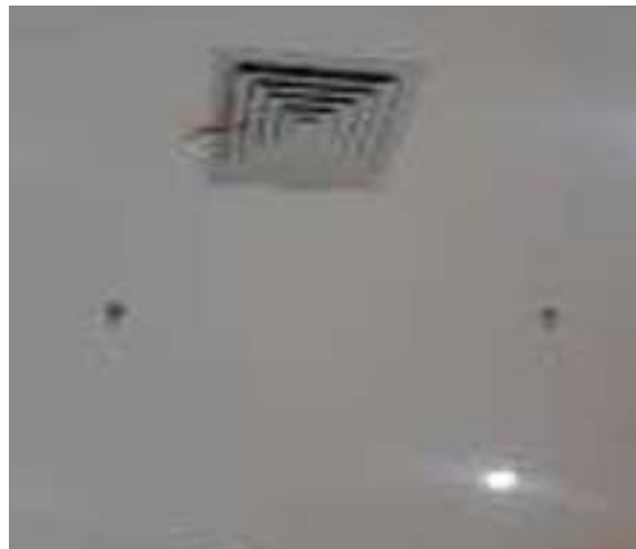
Figure 5:- Fire Sprinkler Protection System.
