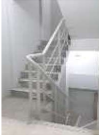
Figure 11:- Life Safety Facility - Emergency Stairs at Lampung City Mall.
