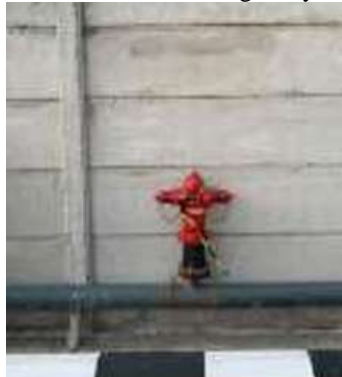
Figure 7:- Hydrant Pillar Fire Protection System Outside LCM Building.
