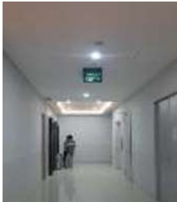
Figure 12:- Life Safety Facility - Exit Signage at Lampung City Mall.
