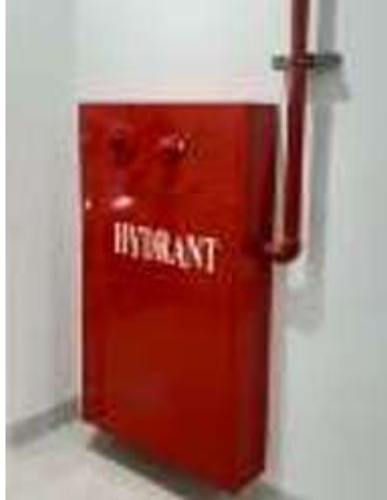
Figure 9:- Fire Protection Hydrant Box Inside LCM Building.
