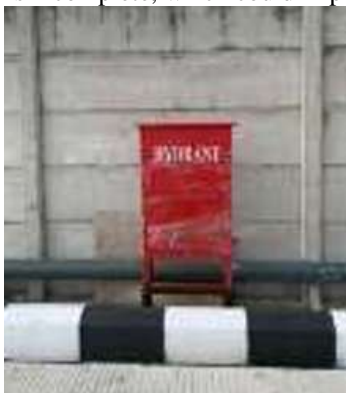
Figure 8:- Fire Protection Hydrant Box Outside LCM Building
