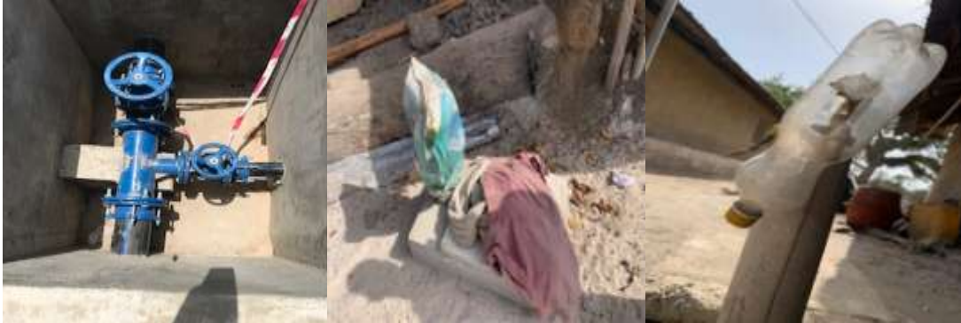
Photo 10:- Drinking water supply and home installation.
