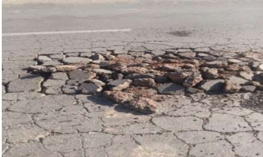
Figure 4:- View of cracking and destruction of pavement.
