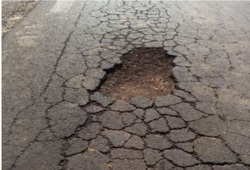
Figure 5:- View of a pothole in the middle of the cracks.
