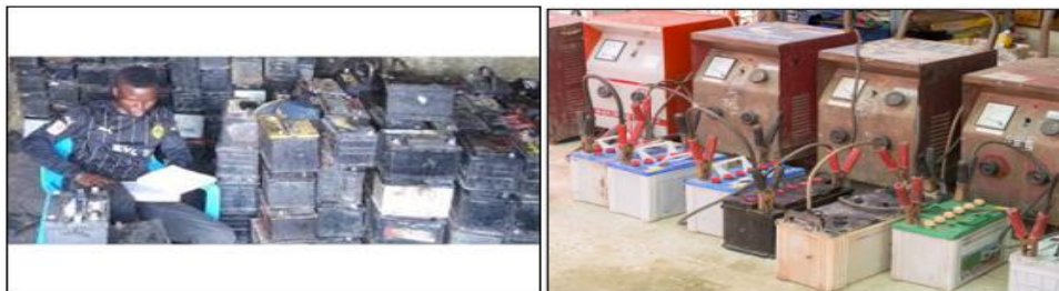
Fig. 4:- The Battery charger (electrolysis).
