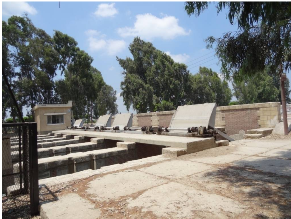
Photo6:- U.S. View ST-7 shows continuing closed two gates
