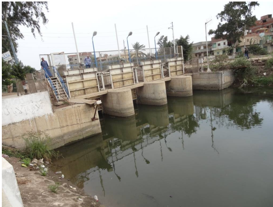
Photo2:- U.S. View of ST-1 shows all gates are fully opened (at W.L. less than the minimum designed W.L.)
