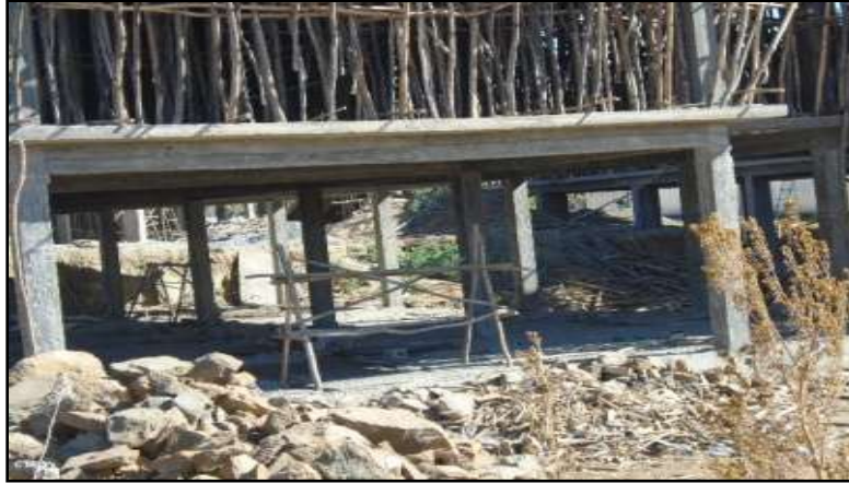
Figure 6:- Visible (4cm) deflection due to small beam Depth.
