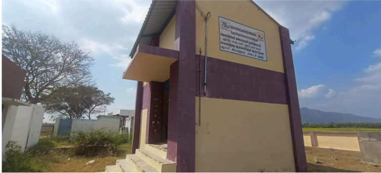
Figure 9 Herbal Unit in Ambalathadi Panchayat, Madurai, lacking locks and proper compound walls for protection.
